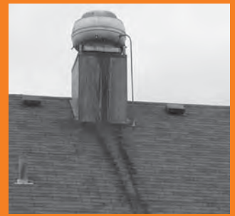
Unattractive Roofs and Fire Hazards
