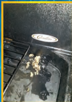
Brush was fully pulled out after 12" and pulled this out of drain tube left in tray.
