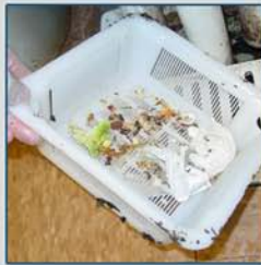
Floor Sink Backups
