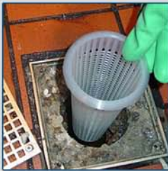
Floor Drain Clogs
